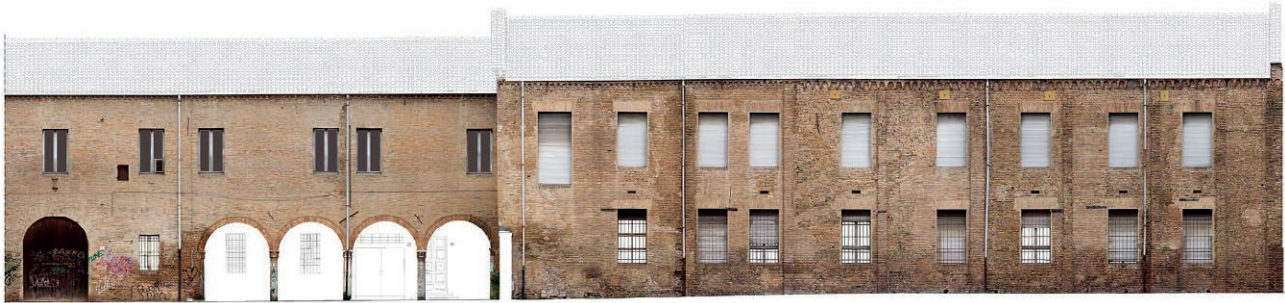
Figure 4. The orthomosaic of the south-facing elevation along Via Roversella, generated in Agisoft Metashape Professional r2.0.10 ® . On the right, the eastern wing reveals substantial structural transformations of the former church's liturgical hall, resulting from its 20th-century conversion into a vocational high school.
