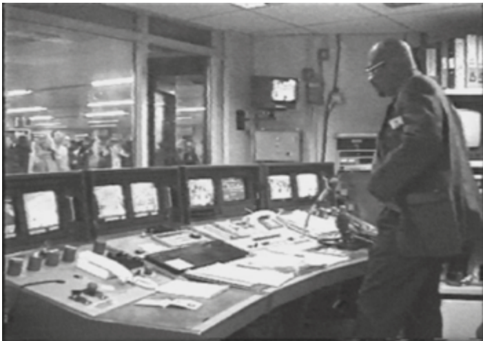
Figure 1: A Station Operations Centre on London Underground
