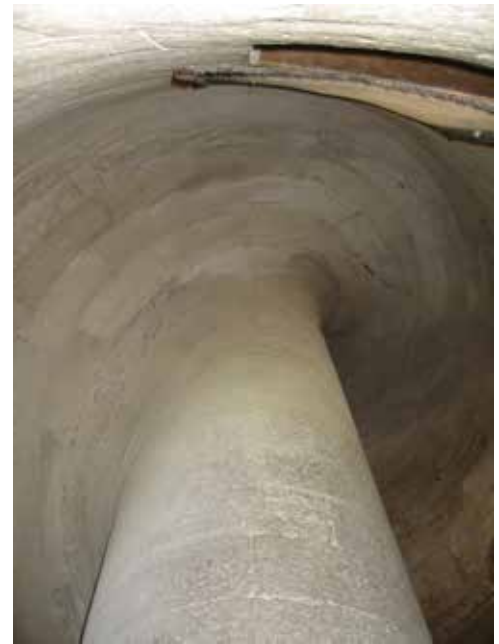
Fig. 10 Abbey church of Saint-Gilles. Remains of the spiral staircase of the destroyed Romanesque choir (photo H. Günther).
